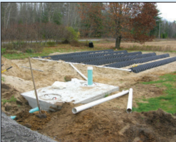
Leaching bed with gravelless trench technology.
